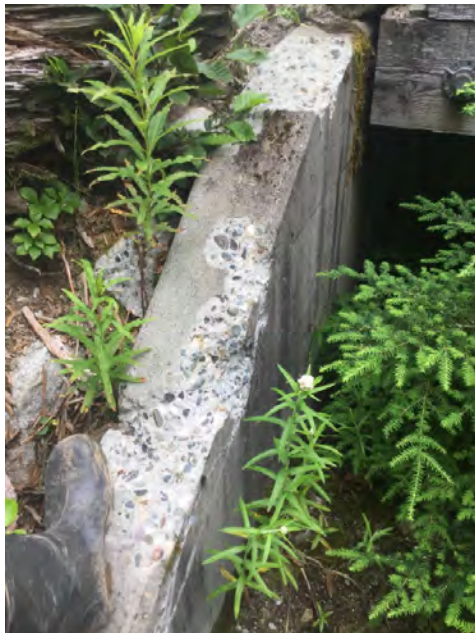
Spall in Left Abutment Upstream Section of Ballast Wall
