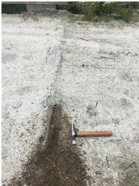
Left Abutment Damaged Ballast Wall
