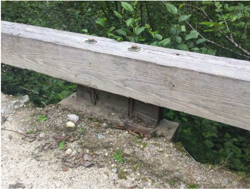
Rotten Guardrail Blocking
